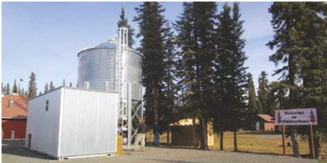
small-scale district heating system
