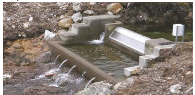
micro-hydro power generation
